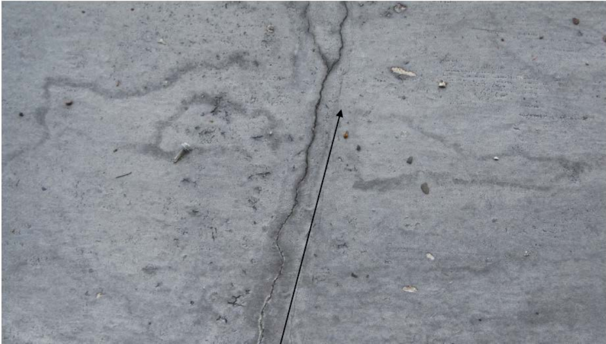
Figure 1 – Existing “Eyebrow” Membrane Splitting on System Administration Building
