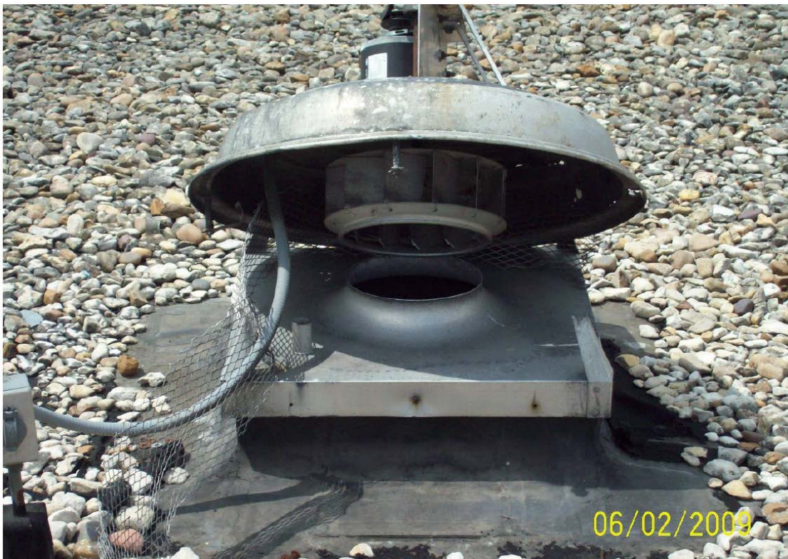
Figure 2 – River Rock Ballasted Membrane Roof with Damaged Equipment
