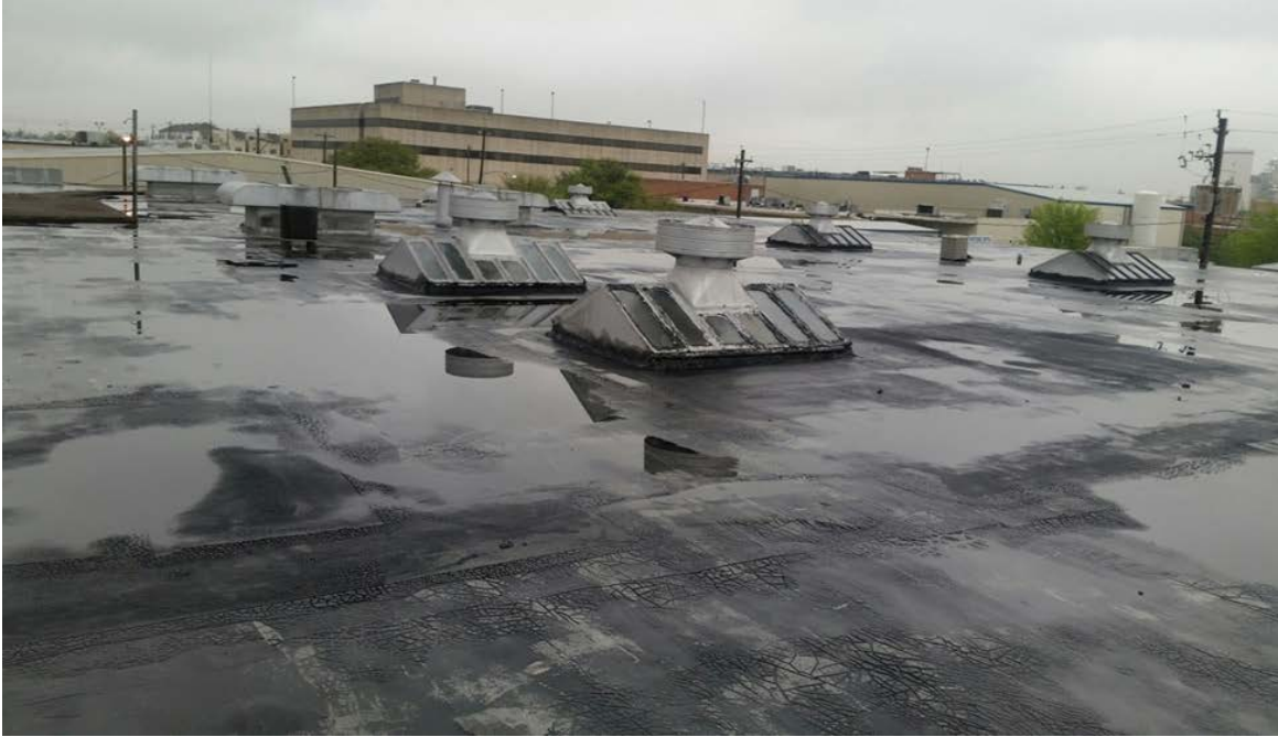
Figure 3 – Distressed Asphalt at Delano Street Warehouse
