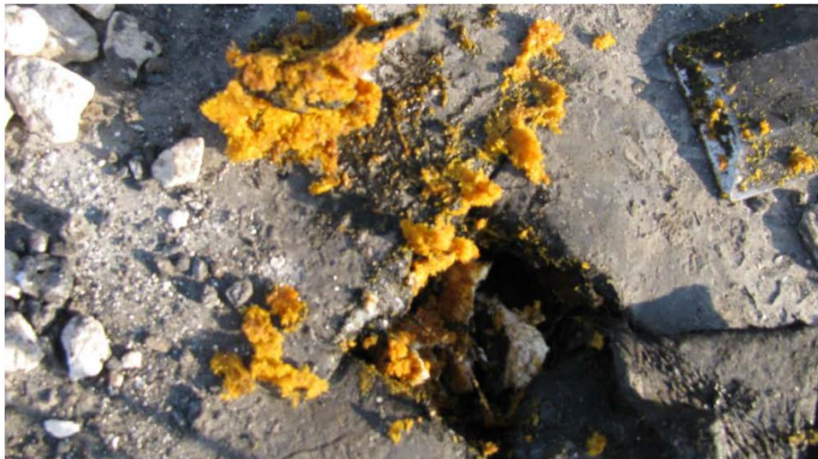
Figure 2 – Evidence of Wet Insulation at J. Don Boney Building
